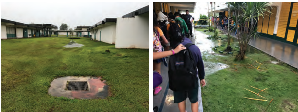
Figure 10: These grass swales do not convey water to the drain inlet or away from the sidewalks and need to be re-constructed.
