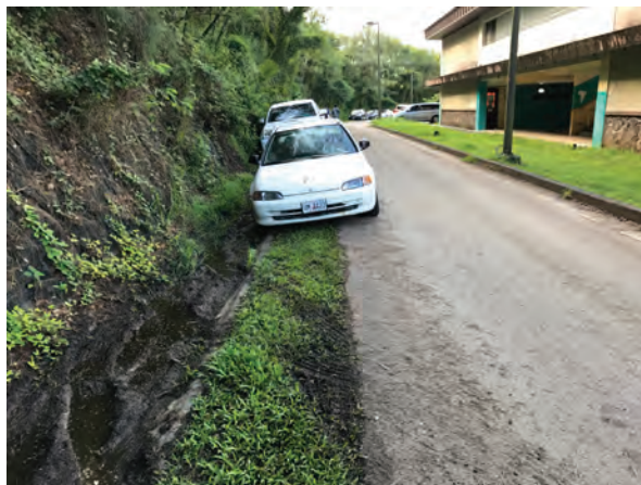
Figure 26: Vehicles parked within a drainage structure damages the planned function of the swale and causes storm water to backup and flood to other areas of campus. These parked cars are also blocking the fire access lane.
