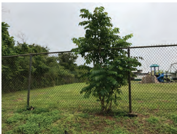
Figure 23: Young tree growing along the fence line will eventually damage the fence unless it is removed soon.
