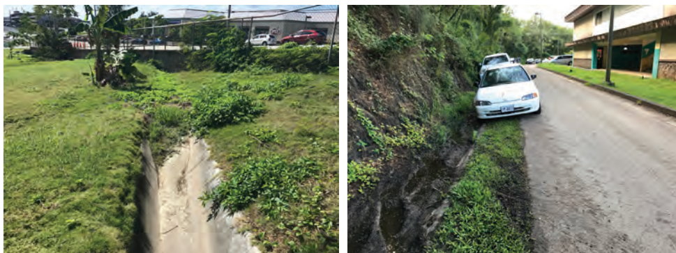
Figure 8: Mud, grass and weeds in concrete and grass swales block the flow of stormwater, causing poor drainage.
