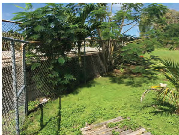
Figure 24: Trees growing along the fence also disrupt the drainage swale and should be removed.
