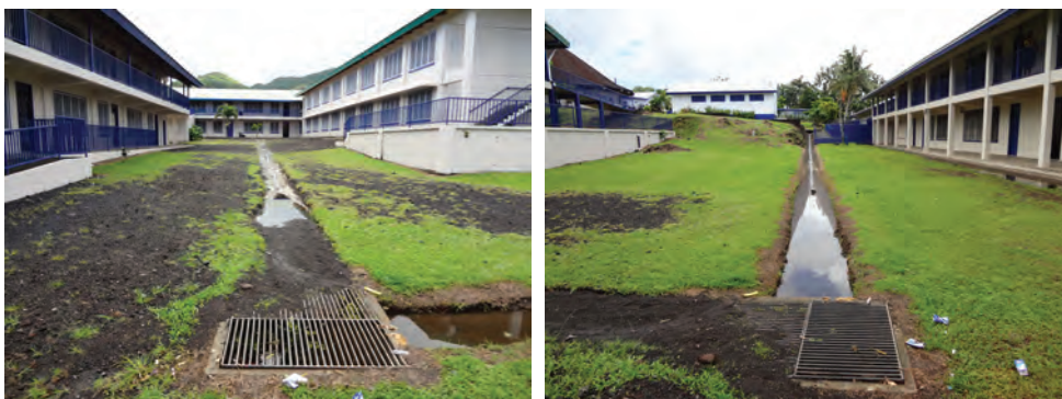
Figure 9: Trench drains are easily clogged with dirt and vegetation. Periodic inspection and cleaning is needed to prevent flooding.
