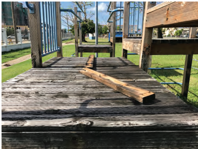
Figure 41: Play structure is compromised by extensive wood rot. Exposed nails are a safety hazard and should be removed immediately. Grass is not a safe surfacing for fall protection; a certified resilient play surface is recommended.
