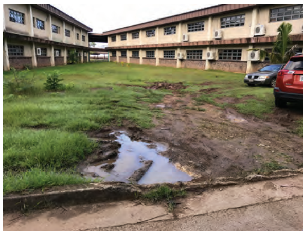
Figure 25: Vehicles parking on grassed areas damages the turf and creates potholes, which degrades site condition, causes erosion, and may create breeding habitat for mosquitoes.
